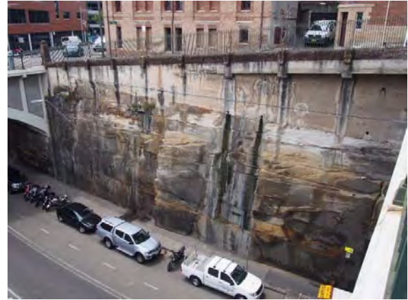
Eastern cut – rough, weathered sandstone cutting with masonry above, with low sandstone walls and palisade fencing at street level
