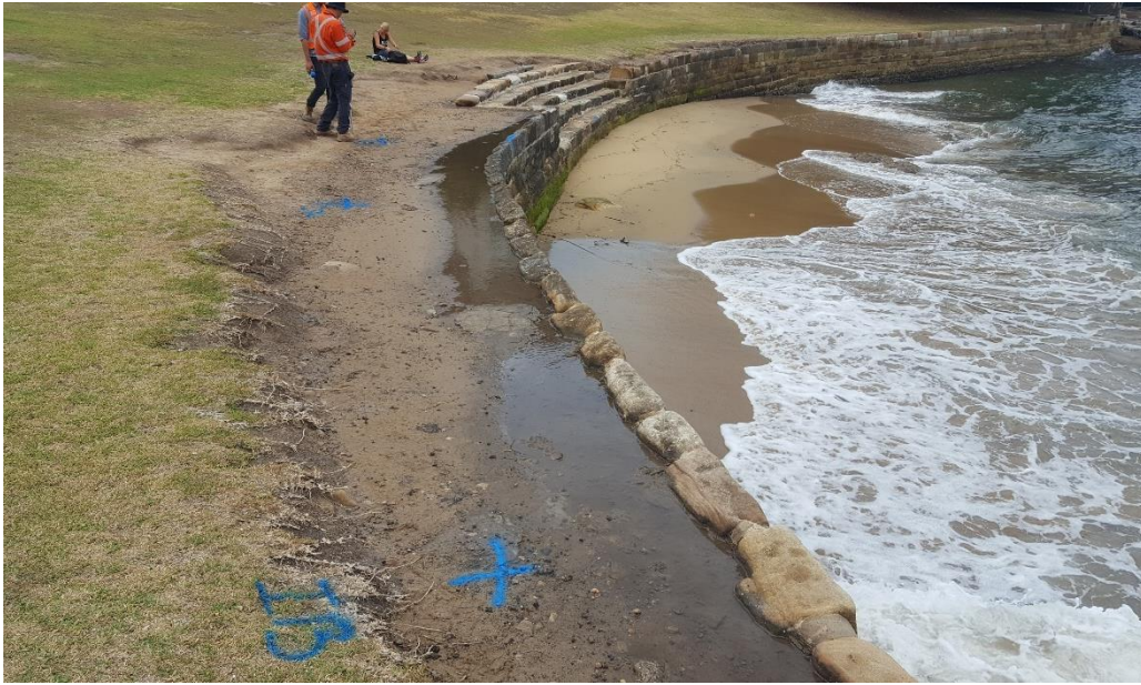
Figure 6: Photograph of the seawall showing the approximate location of the proposed ramp. The steps are in the background. Supplied by Andreas Mindt, Project Manager, JHCPBG, taken 20/12/2017.
