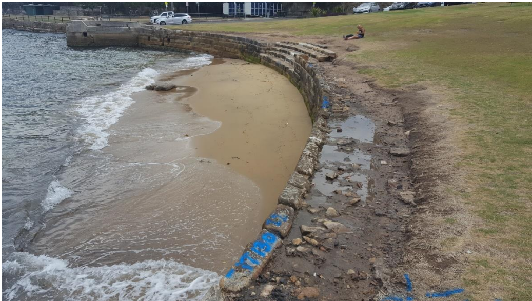
Figure 7: Photograph of the seawall showing the approximate location of the proposed ramp to the immediate left of the steps. Supplied by Andreas Mindt, Project Manager, JHCPBG, taken 20/12/2017
