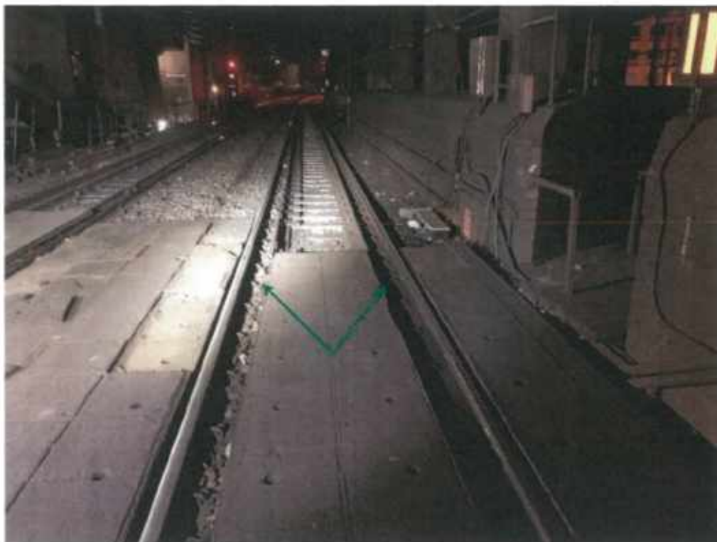
Plate 3: Up city inner, potential pinch points. 12 meters of tiles that need to be replaced as part of the pad.
