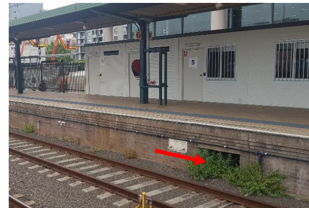
FIGURE 2.7: EXISTING OPENING, IDENTIFIED BY RED ARROW, PROVIDING ACCESS TO THE CAVITY WITHIN THE EXTENDED SECTION OF PLATFORM 1.
