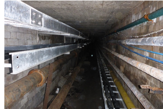
FIGURE 2.46: TYPICAL VIEW WITHIN WATER MAIN TUNNEL SHOWING SOME OF THE MAIN FEATURES AND EXISTING SERVICES. SOURCE: SAS TTI JOINT VENTURE
