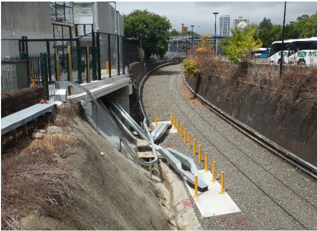
FIGURE 2.19: VIEW SOUTH ALONG DARLING HARBOUR. NOTE SHOTCRETE ON EASTERN EMBANKMENT IN THE FOREGROUND AND EXISTING TRANSITION OF SERVICES INTO THE DIVE.
