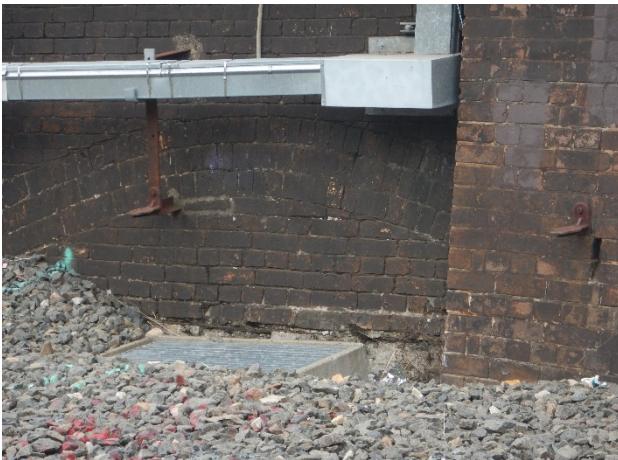
FIGURE 2.22: BRICK CULVERT, BRACKETS AND SYDNEY TRAINS SERVICES PRESENT ON EAST EMBANKMENT WALLS.
