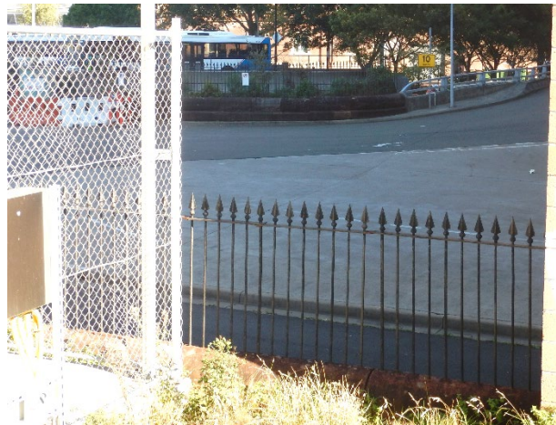
FIGURE 2.14: DETAIL VIEW OF THE WESTERN BOUNDARY FENCE ADJACENT TO PLATFORM 1 (FOREGROUND) EXTENDING AROUND THE DHGL IN THE BACKGROUND.
