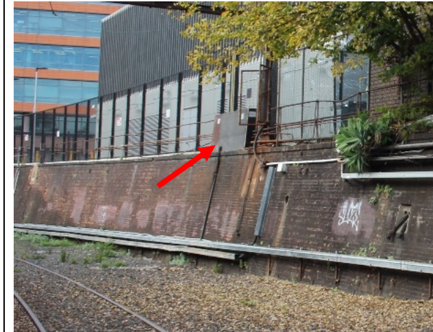
FIGURE 2.31: CURRENT VIEW, INDICATIVELY SHOWN BY RED ARROW, OF THE LOCATION WHERE SERVICES WILL BE TRANSITIONED INTO THE DIVE.
