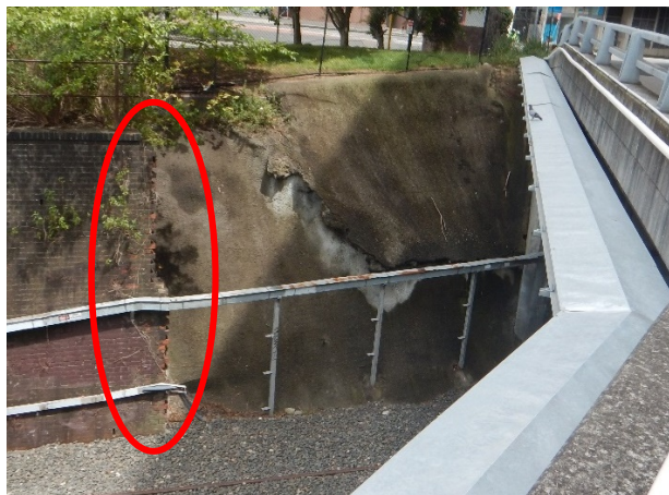
FIGURE 2.23: EXPOSED EDGE OF WESTERN BRICK EMBANKMENT WALL (OUTLINED) INDICATING REMOVAL OF ORIGINAL FABRIC WHERE SHOTCRETE HAS BEEN APPLIED.
