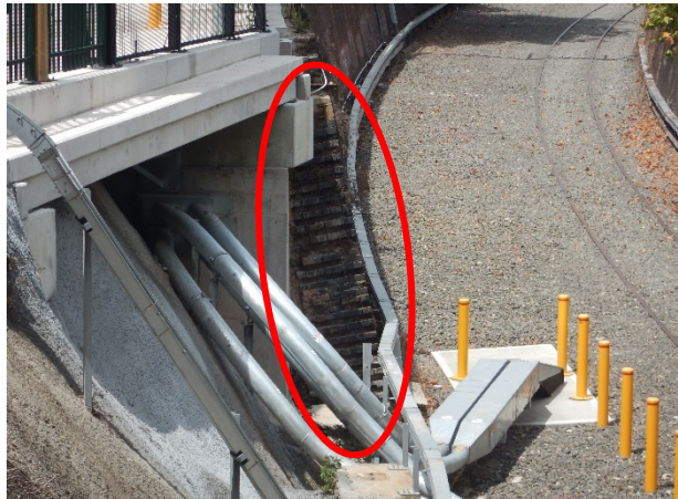
FIGURE 2.20: DETAIL OF EASTERN EMBANKMENT SHOWING THE EXPOSED END OF THE 1926 BRICKWORK (OUTLINED) FOLLOWING MODIFICATION OF THE EMBANKMENT.
