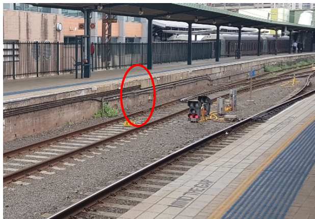
FIGURE 2.6: JOINT IN WALL OF PLATFORM 1 WHERE PLATFORM HAS BEEN EXTENDED TO THE SOUTH.
