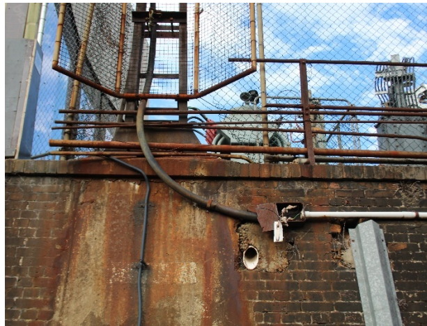
FIGURE 2.26: EXAMPLES OF EXISTING INTRUSIVE INTERVENTIONS TO THE EASTERN WALL OF THE DHGL, INCLUDING PIPEWORK, FIXTURES, REMOVAL OF BRICKWORK AND CONCRETE PATCHES. NOTE REMNANT SECTION OF FOLDED METAL BALUSTRADE ON THIS SECTION OF WALL.
