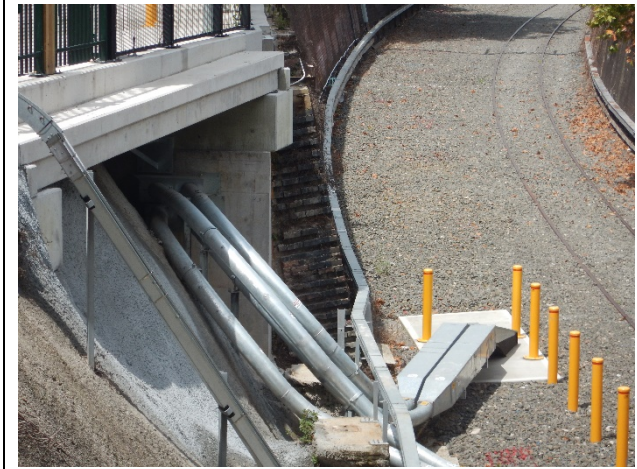
FIGURE 2.27: EXISTING GST AND CABLE TRANSITIONS FOR SYDNEY TRAINS SERVICES ON THE EASTERN EMBANKMENT BELOW EXISTING REINFORCED CONCRETE BEAM.
