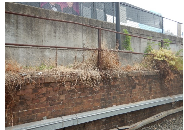
FIGURE 2.24: DETAIL VIEW SHOWING ORIGINAL PIPE RAIL AND FOLDED METAL BALUSTRADE ON THE WESTERN WALL. BEYOND IS THE CONCRETE BOUNDARY WALL OF THE BUS DEPOT, WHICH IS NOT PART OF THE CENTRAL STATION SITE.
