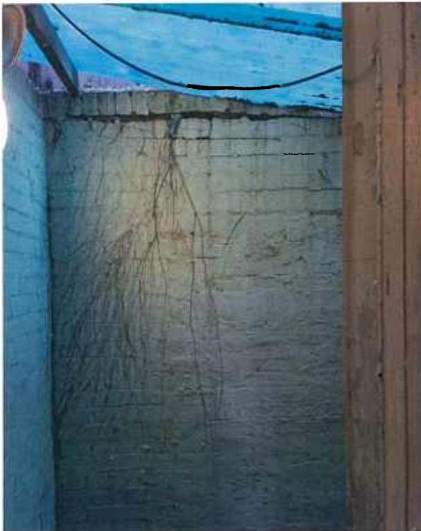
Photo of rear back wall to male toilet
