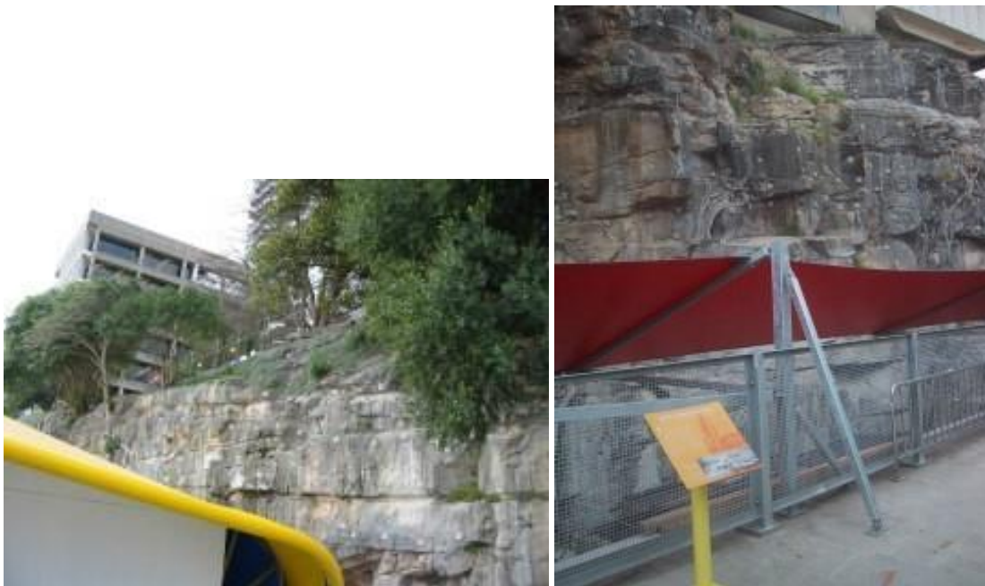
Figure 4.30 Rock bolting of the sandstone cliff, Site C, Luna Park undertaken prior to 2006 (OCP 2006:23).
