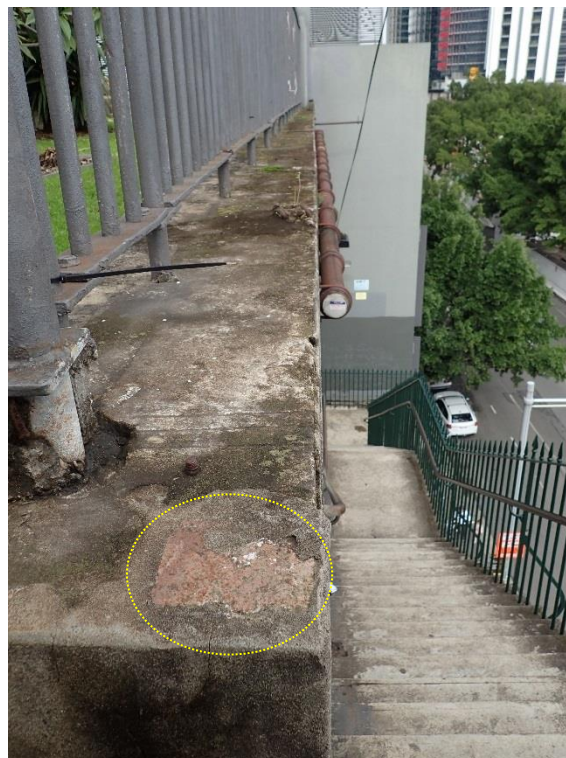
Figure 4.9 View down the upper flights of steps from High Street. Note eroded render exposing what appears to be a brick.
