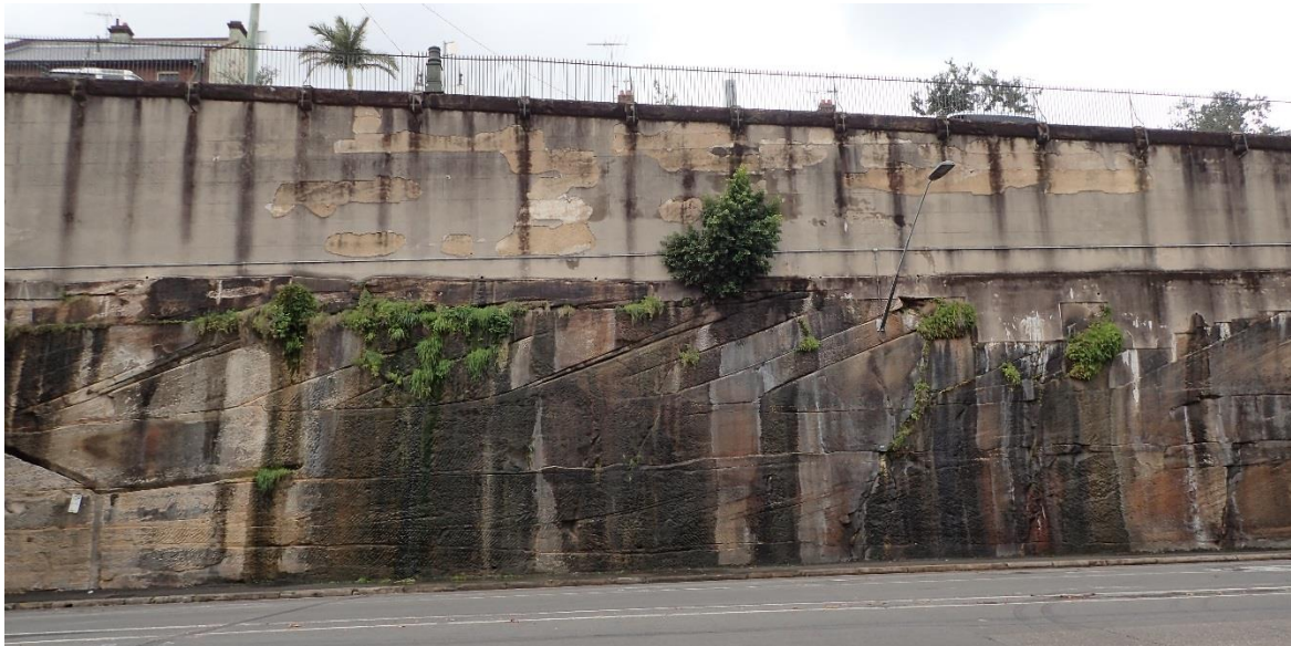
Figure 4.18 A series of modern lights attached to the wall and cutting with attached signs Supplied from meter panel/for outages call City of Sydney 1300 651 301 . Note the colonising grasses and ferns, and the stratigraphic layering of the bedrock.
