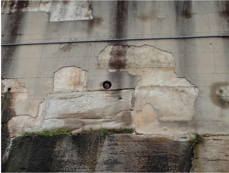
Figure 4.13 A section of the cutting and wall. The render is scored to replicate masonry blocks and is aligned along the line of the natural bedrock, above which the underlying sandstone blocks have been exposed. Note, the weep hole has been colonised by a pigeon.
