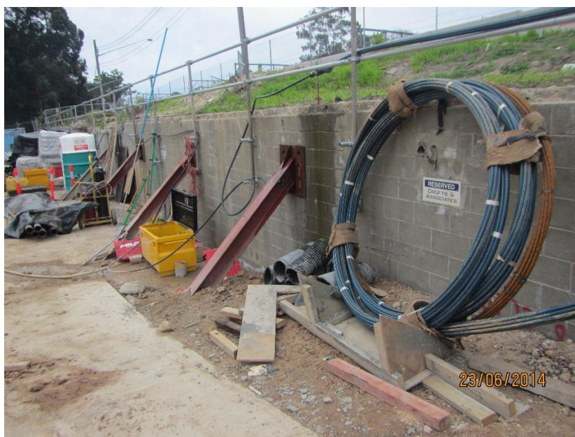
Figure 4.28 An example of retaining props, albeit at a much smaller scale than would be required for the High Street cutting (JHCPBG).
