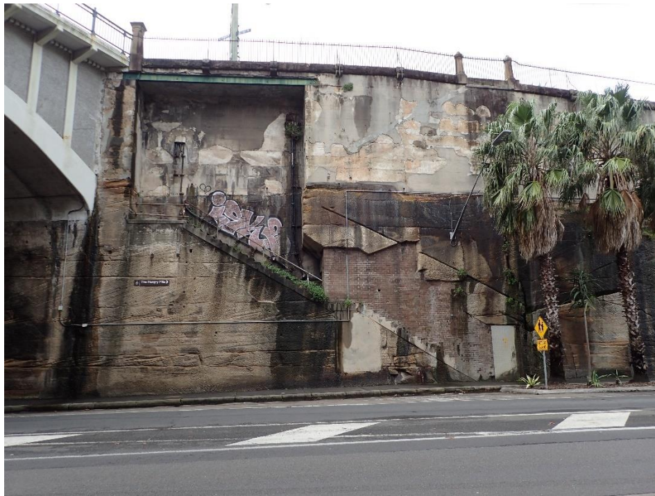
Figure 4.6 View east to the Hickson Steps. Note the brick infill rendering the steps unusable. The sign, left, identifies 'The Hungry Mile' and the steel door to the right identifies buried RailCorp electrical cables.
