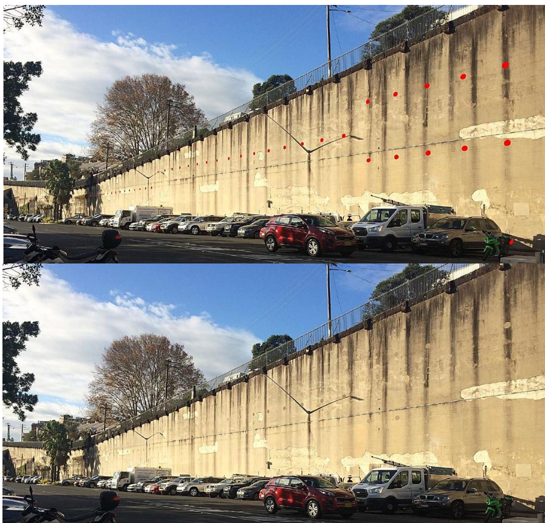
Figure 4.34 Photomontage of the appearance of the retention anchors following patching. The image above shows the locations in red, while the image below is the after patching appearance (JHCPBG Appendix D).
