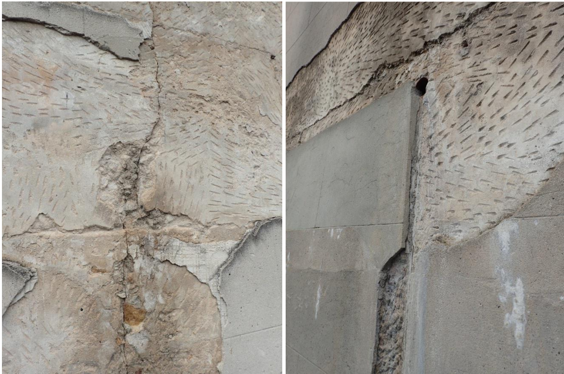
Figure 4.15 Exposed patches of render indicate that at least some sections have three layers of render and the lower layers are pecked to create a rough surface for the next layer (left). Drainage channels have been shaped into the render below the original weepholes (right).
