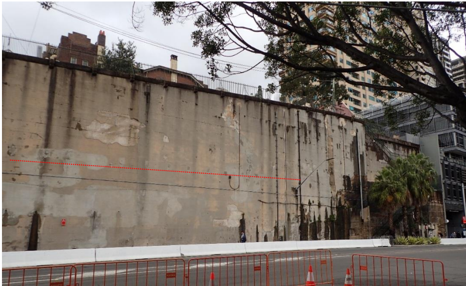
Figure 4.2 View south-east where a greater quantity of the natural sandstone has been removed. A line of the 1995 anchors is indicated.
