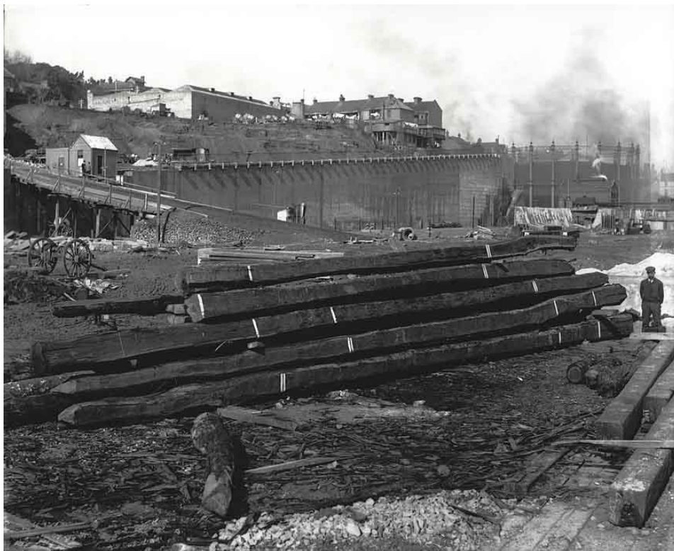
Figure 4.21 Photograph of the construction of Hickson Road showing what appears to be the overbridge which later linked High Street with the Darling Harbour wharves. Also note the mounds of fill above the wall ( https://s3-ap-southeast-2.amazonaws.com/srns-public-photos/9856_a017_A01700025.jpg ).
