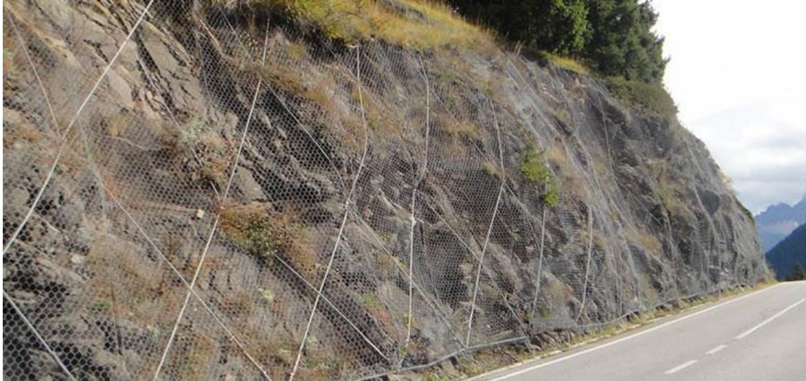
Figure 4.35 Protective netting attached to a road embankment (JHCPBG).
