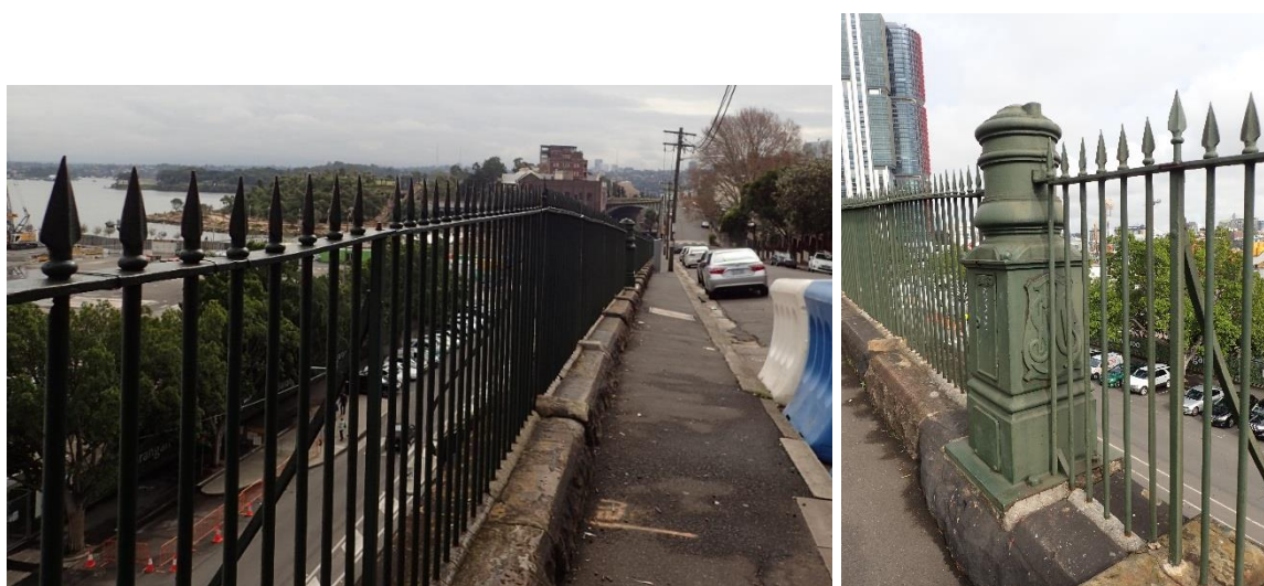
Figure 4.5 View north along the palisade fence (left), and detail of one of the cast iron posts supporting the fence. The fence is concreted into sandstone coping.
