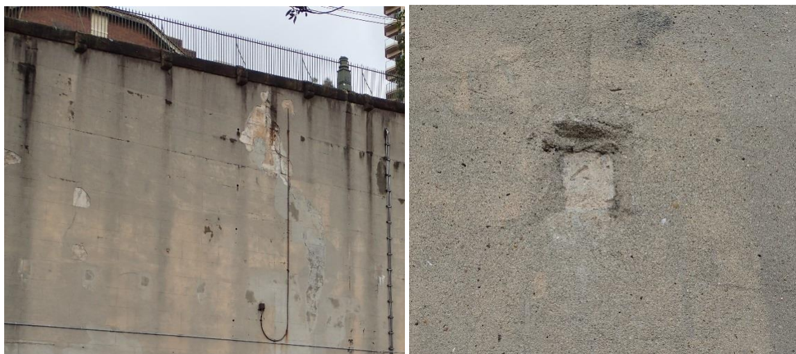
Figure 4.33 1995 retention anchors along a section of the High Street retaining wall (left), and a detail of the recessed and patched anchor.
