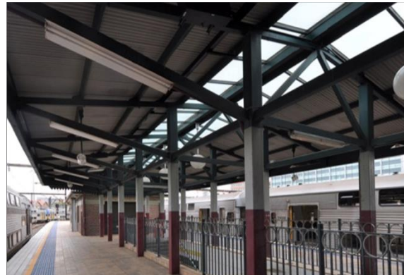
Figure 3: Typical awning extension on the Sydney Terminal platforms and extant balustrading (Source: Rappoport, 2013).
