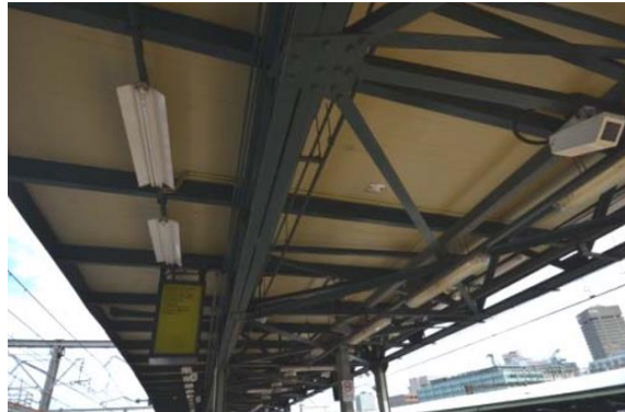
Figure 5: The steel trusses and reinforced concrete awning along the platforms (Source: Rappoport, 2013).
