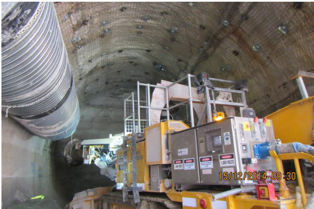
Figure 7: Roadheader as used for construction of cross passage on recently completed Sydney Metro Northwest project. Note additional working room required in comparison to small excavator (Brokk).
