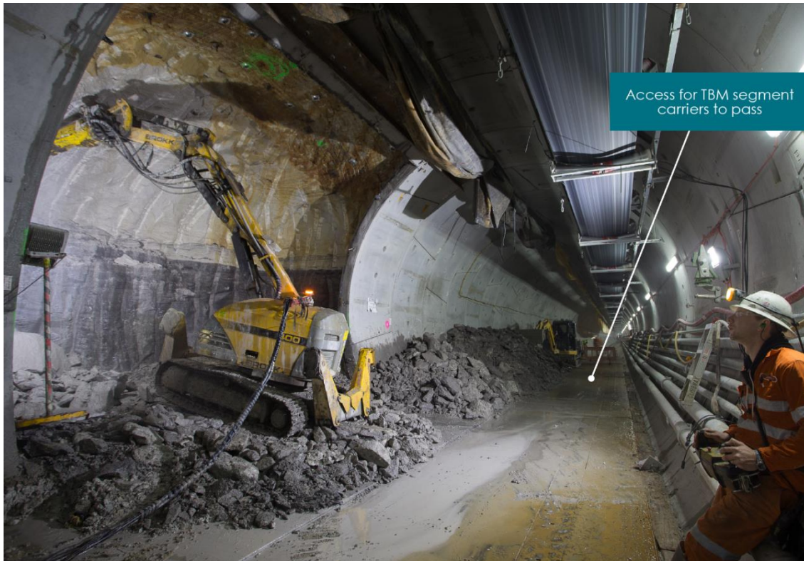
Figure 5: Cross passage excavation using small excavator (Brokk). Note constrained working area due to requirement to maintain through traffic.
