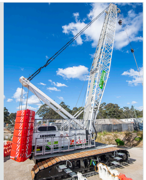
The electric crane in operation at the Claremont Meadows Services Facility site.
