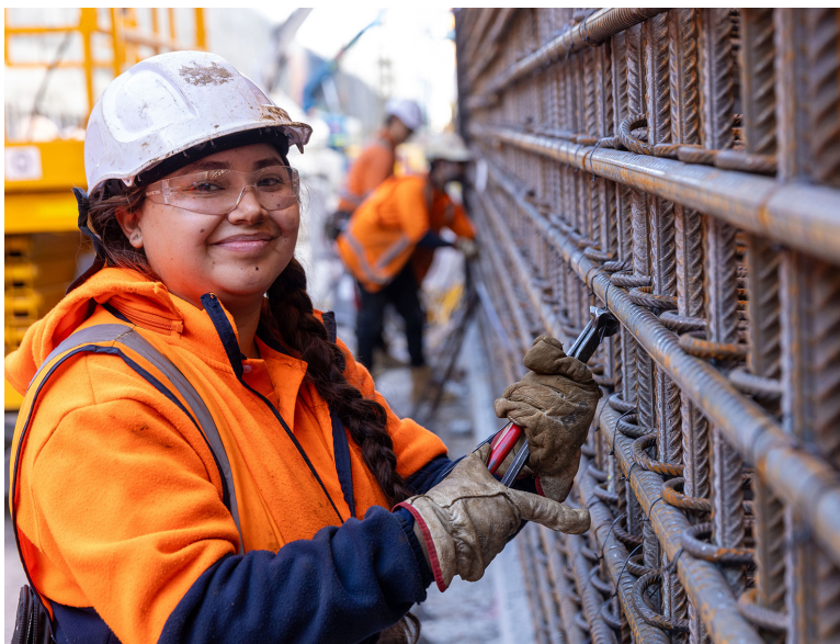
The team is progressing with concrete pours for the base slab and walls at all station sites.
