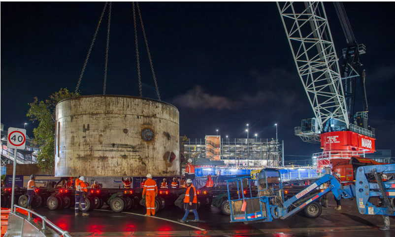
A TBM shield is lifted onto a truck at the St Marys Metro Station site.
