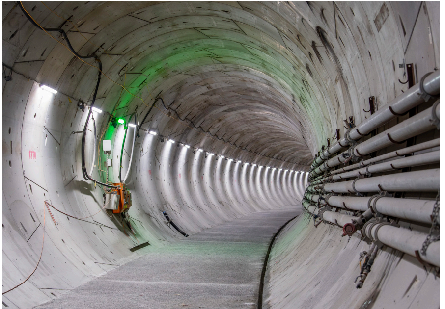
One of the tunnels between Airport Terminal Station and Bradfield Station with a floor ready for the metro rail tracks to be installed.
