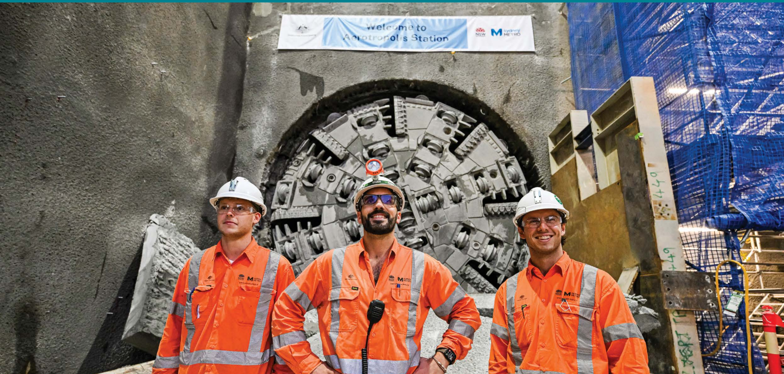
TBM Eileen was the first TBM to break through at Bradfield late May 2024.
