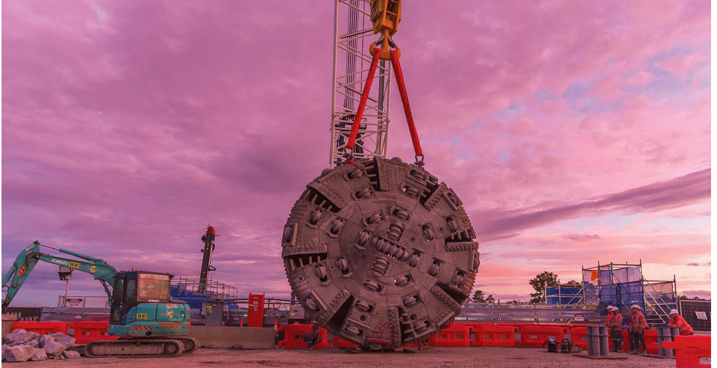
TBM Eileen's cutterhead is lifted off the front shield and out of the station box.
