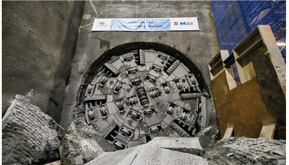
TBM Eileen broke through at the Bradfield Station site in late May.
