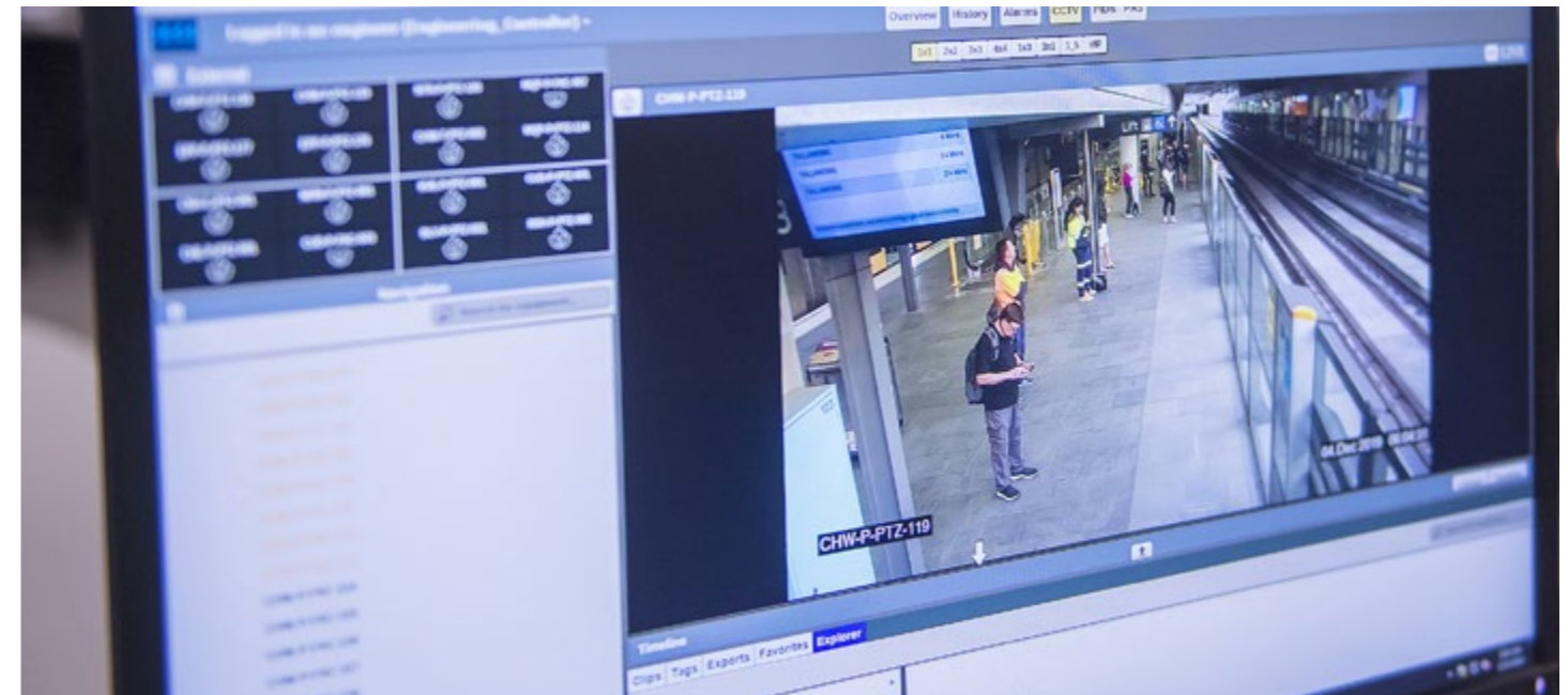
Expert train controllers work in a state-of-the-art Operations Control Centre at Tallawong.
