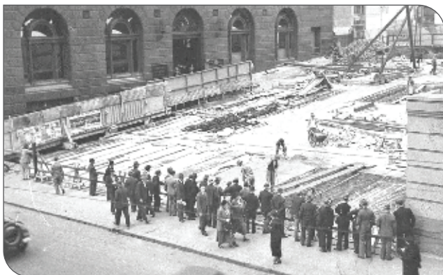
Forming the Martin Place roadway between Castlereagh and Elizabeth Streets, c193. Source: SLNSW hood_01073
