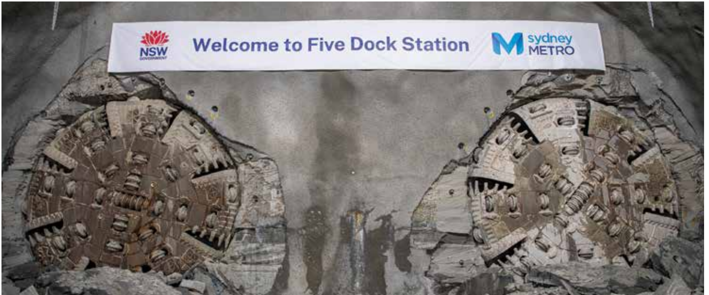
Two tunnel boring machines (TBMs) have achieved a double breakthrough at Five Dock Station.
