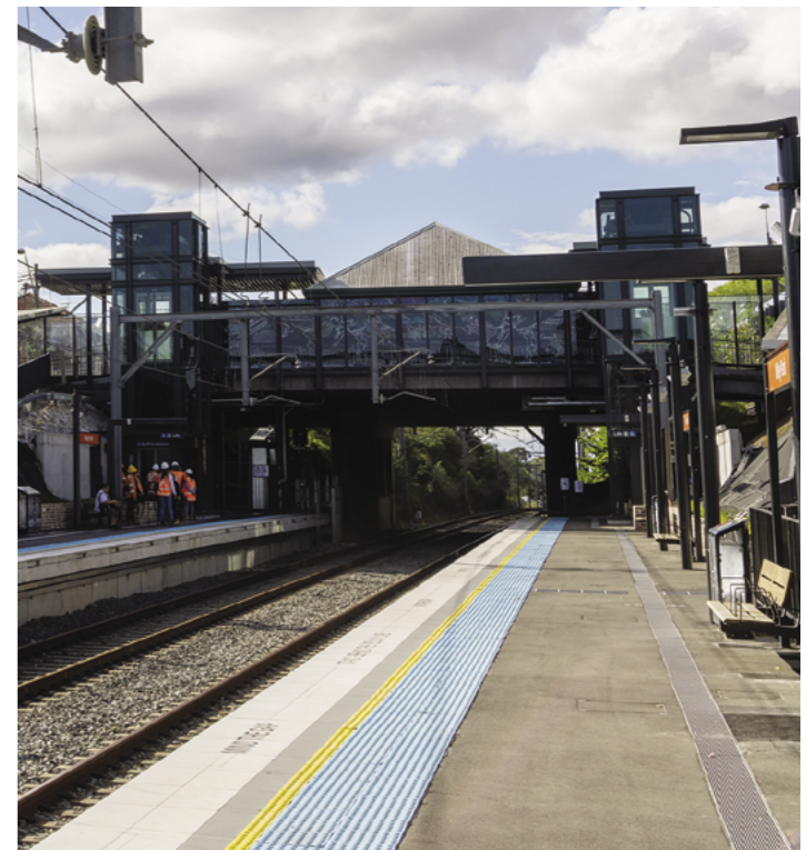
New lifts at Wiley Park Station are now in operation.
