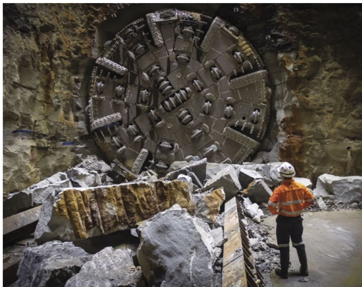
TBM 3 Wendy, dug a 6.2-kilometre tunnel to the edge of Sydney Harbour, on the City & Southwest project.
